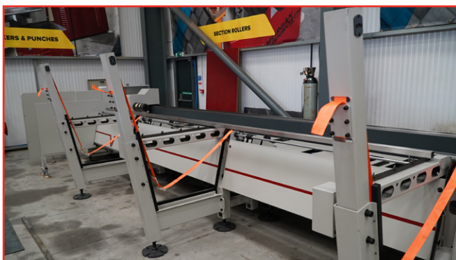
DUAL LOADING SYSTEMS
