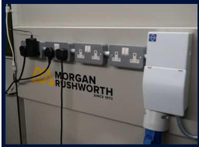
Integrated Electrical Panel & Fuseboard
